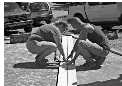
Trish and Jason Scott mark out a wall for their new home.
